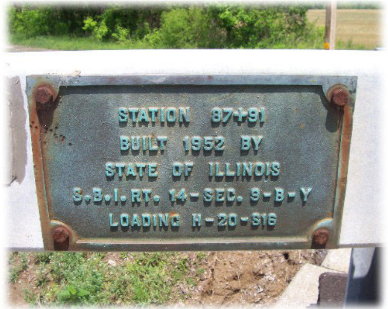
Note: somewhere on every bridge is a plaque showing when it was constructed.
