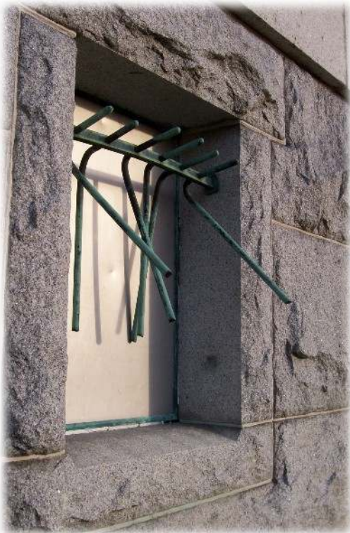
Evidence of past vandalism.
