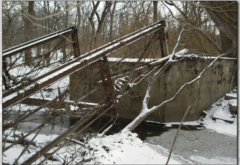
Axeman's Bridge recently collapsed.
