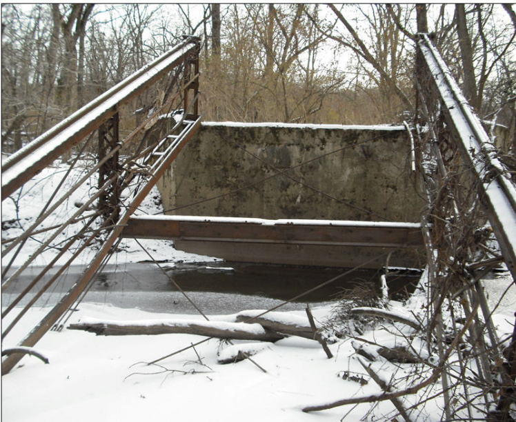
This simple, iron bridge could not withstand the test of time.
