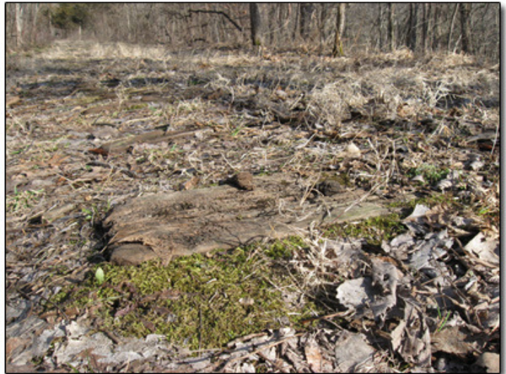
Nature has reclaimed much of the old rail bed, but railroad ties can still be seen sticking out of the grass.
