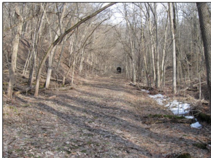
A long trail ends at one entrance to this abandoned railroad tunnel. The opposite entrance is buried by debris.
