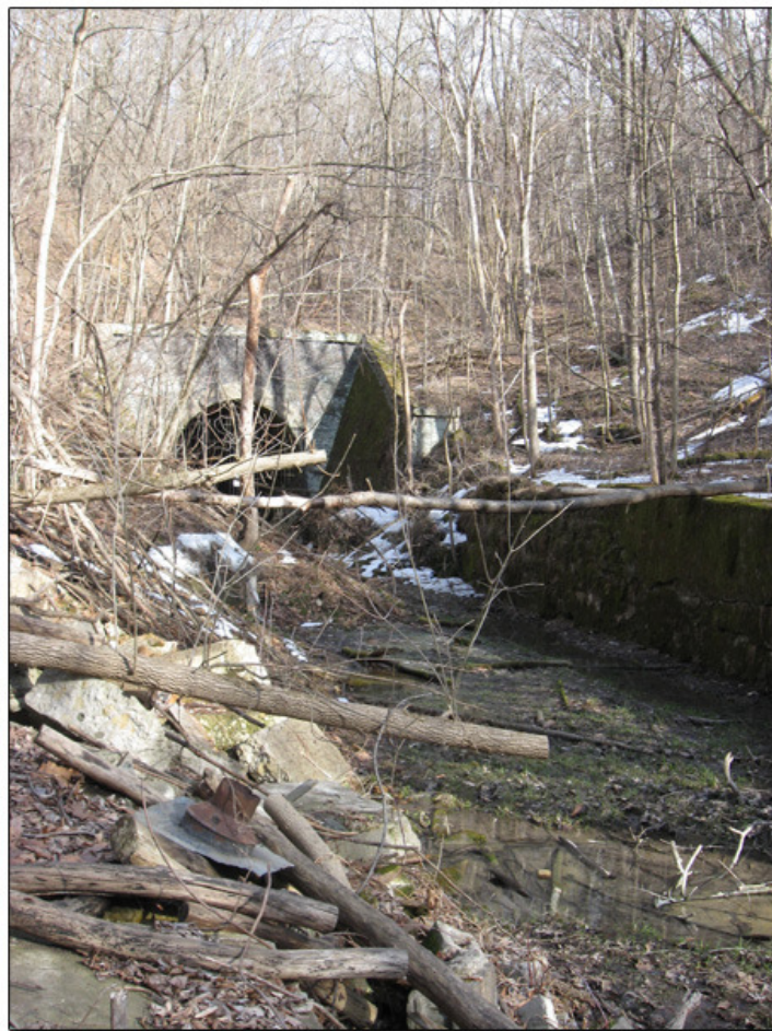
Near the tunnel, the sides of the former rail bed become steep and covered with dangerous debris.
